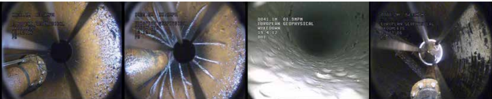
Rising main joint in 600mm id plain steel lined borehole
